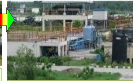
Zero discharge Plant. In-house ETP and STP plants
